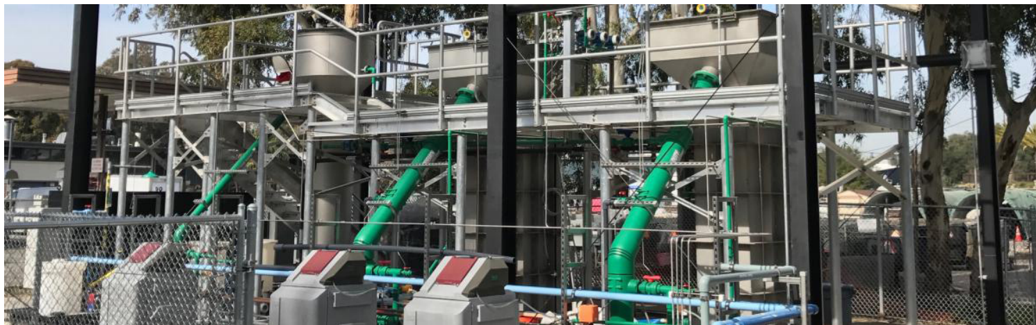
The William and Cloy Codiga Resource Recovery Center (CR2C)
